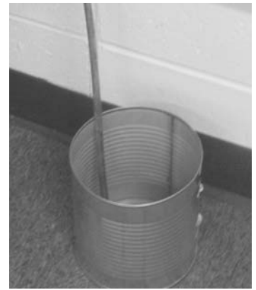
Buckets are used to stop rain water from dripping on floors of the cafeteria and several classrooms at Hamilton Bicentennial Elementary School. The proposed Capital Projects referendum would replace deteriorating roofs at both elementary schools and the High School.
